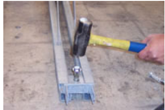
6. Gently hammer bolt into the hole until bolt head & washer are firmly seated against anchor plate.
